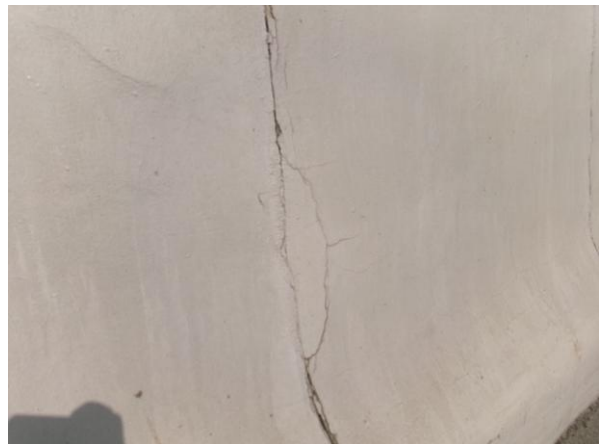
S3 방호벽 들뜸(0.1×0.4m)
